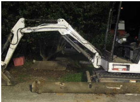
(L) Section of badly deteriorated pipeline that caused the De Solo main break. (R) Repaired De Solo pipeline.
