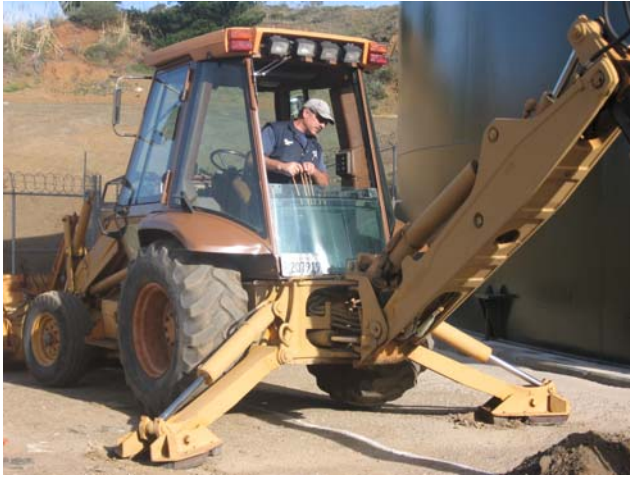
Frank Capizano excavating for electrical / SCADA system improvements for New Royce Tank.
