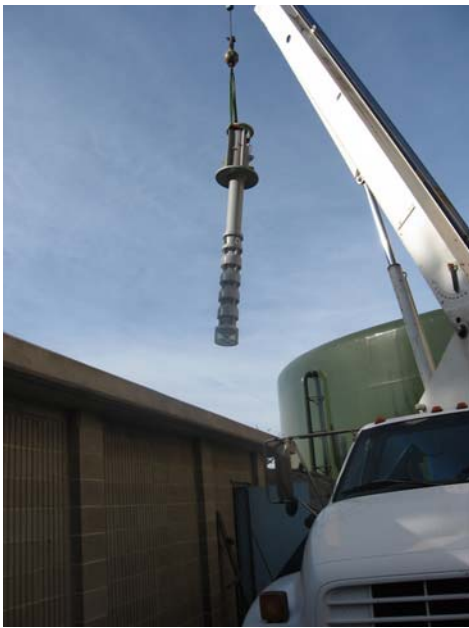
New Pump at Royce Pump Station. (Left & Right)
