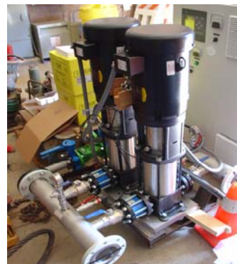
Booster pump awaiting installation.
