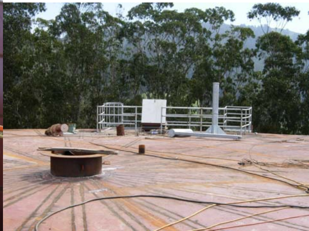
(Right) Gypsy Hill Tank Roof Access Platform with Roof Hatch + Roof Crane
