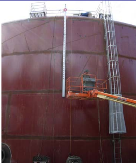
(Left) Gypsy Hill Tank: Safety Ladder + Roof Access Platform
