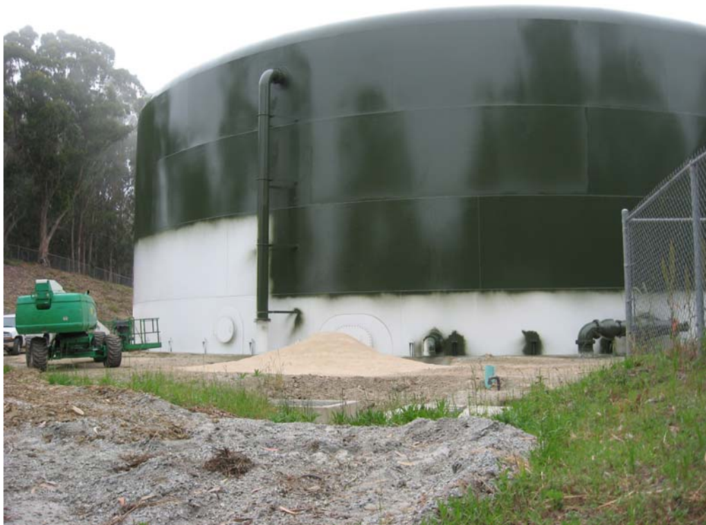
Photo 2: New three million gallon potable water tank at NCCWD's Gypsy Hill site (TRA, June 2007)
